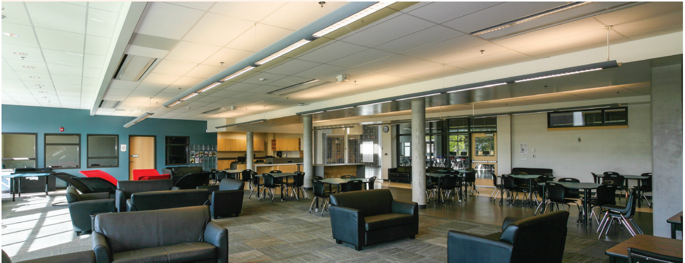
Titus CBAL-24 active chilled beams installed in Steinbach School, Manitoba
