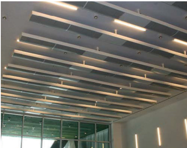
Exposed passive chilled beams installed in a lounge area
