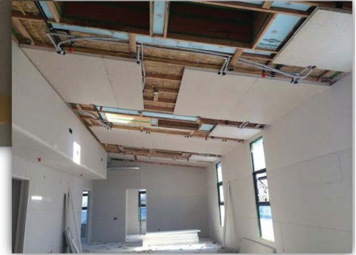
Installation of radiant cooling panels. Note the high number of water connections required for the system.
