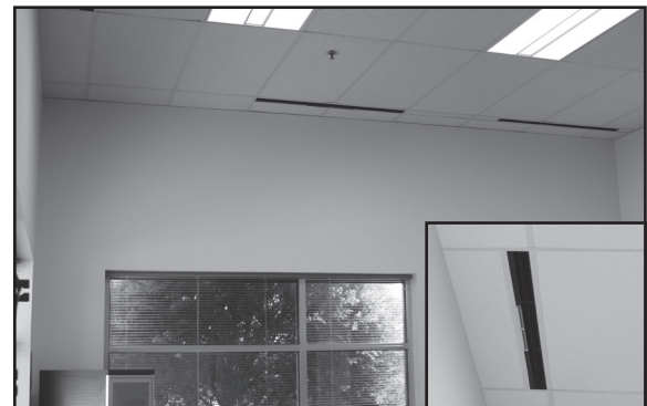
Below: EOS Primary-Secondary (DR) configuration installed in an office environment along the perimeter
