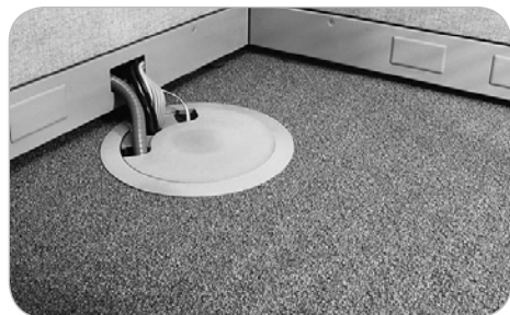
TAF-G diffuser installed in the floor of an office cubicle
