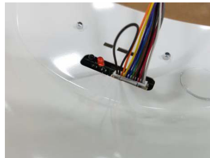
Figure 3. Control board wiring connection
