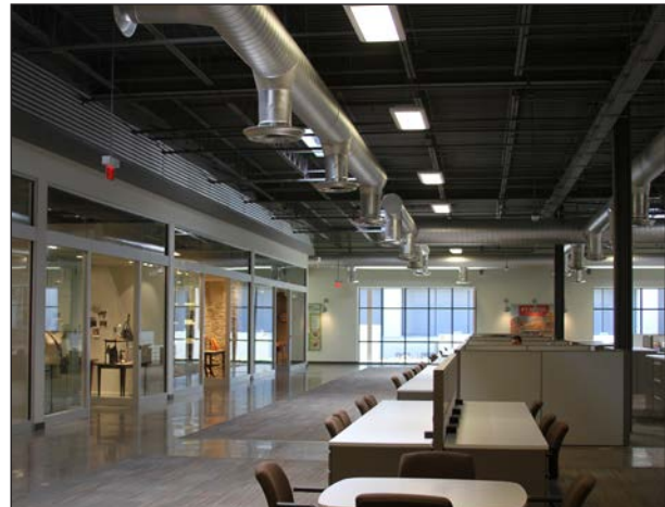
TMRA-AA installed in an office environment
