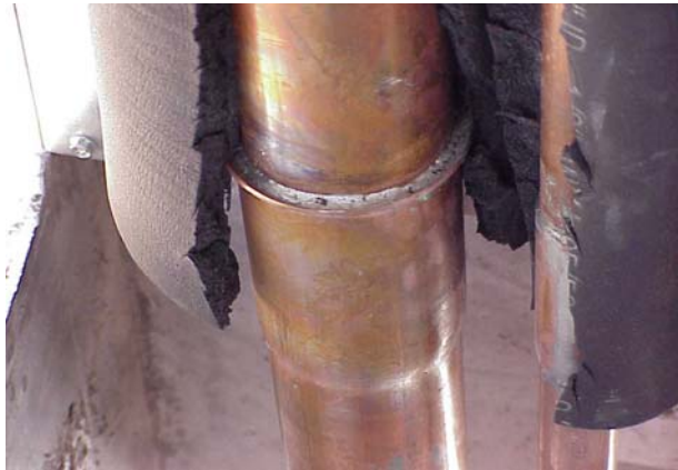
Correctly soldered extension joint
