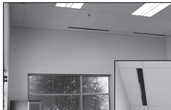
Below: EOS Master-Drone (DR) configuration installed in an office environment along the perimeter
