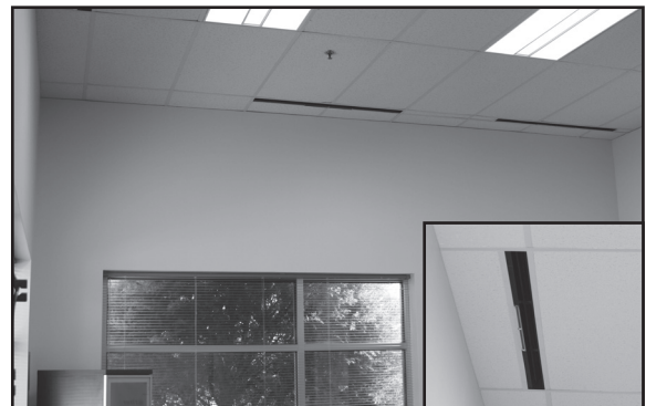
Below: EOS Primary-Secondary (DR) configuration installed in an office environment along the perimeter
